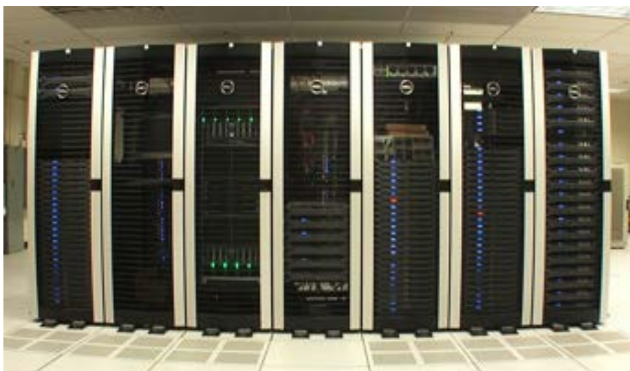
A cluster of Dell computers at FNMOC in 2011. Source: NPS Video Portal
