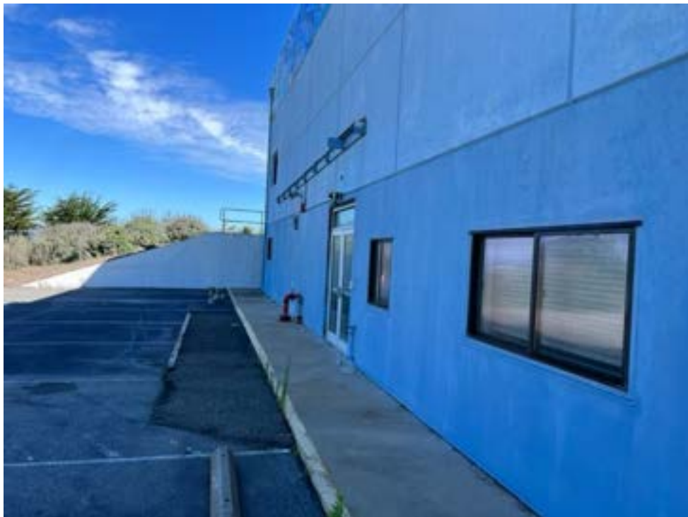
Photograph 8: View looking north at the west side of the building towards the rear.
